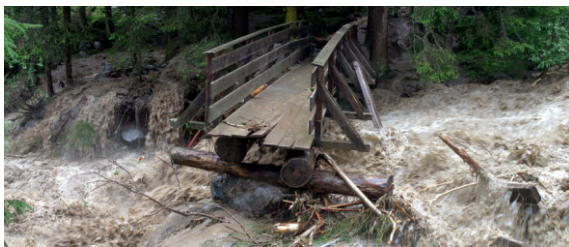
Figure E6.6: Flooding in a mountain stream in the Ötztal in August 2006 (photo M. Weber).
